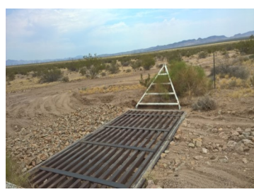
Photo of cattle guard repair. Cattle guards are used on the BCCE to prevent tortoises from crossing into the road.
